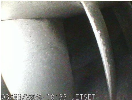
Inlet Coating Loss
