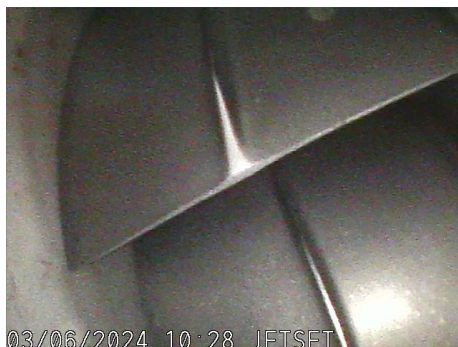
Low Compressor (Fan)
