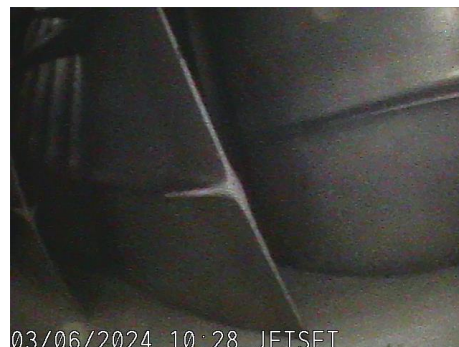
Low Compressor (Fan)
