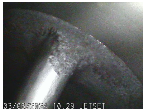
Inlet Coating Loss
