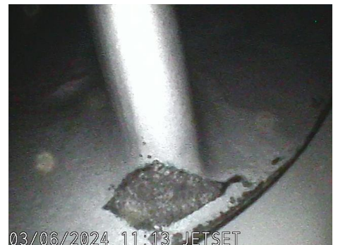
Inlet Coating Loss
