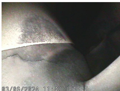
HT Vane Outer Wall Crack
