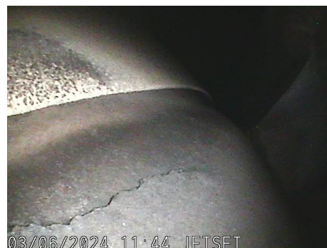
HT Vane Outer Wall Crack
